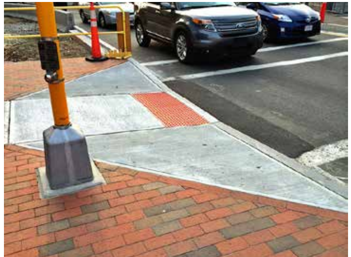
Image: Curb cuts that are ADA compliant. (Source: Unit Boston)
